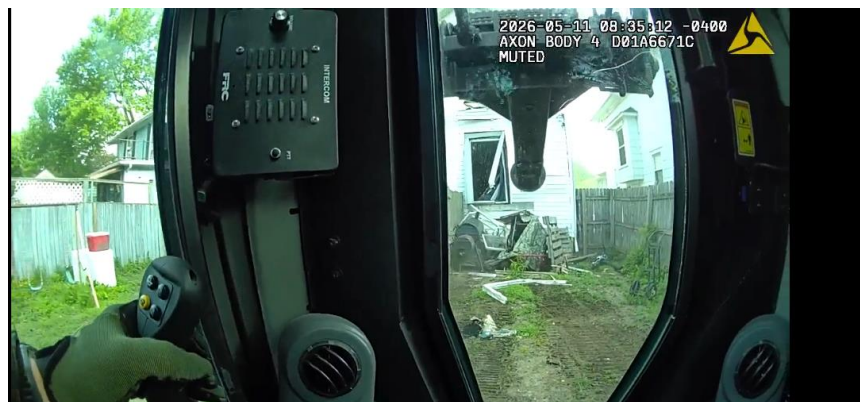
Figure 4: Damage to Rear Wall of Home
