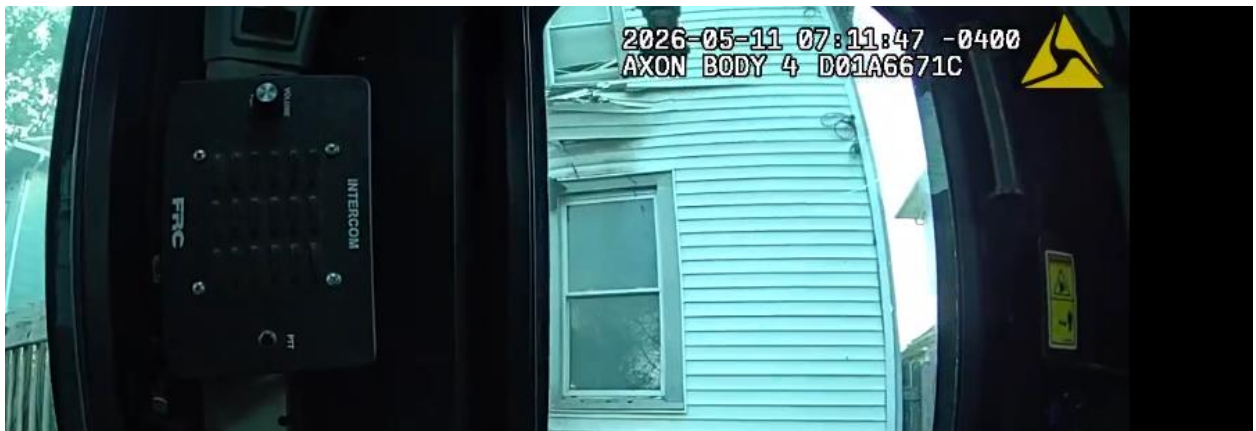
Figure 2: Damage to Second Floor Wall.
