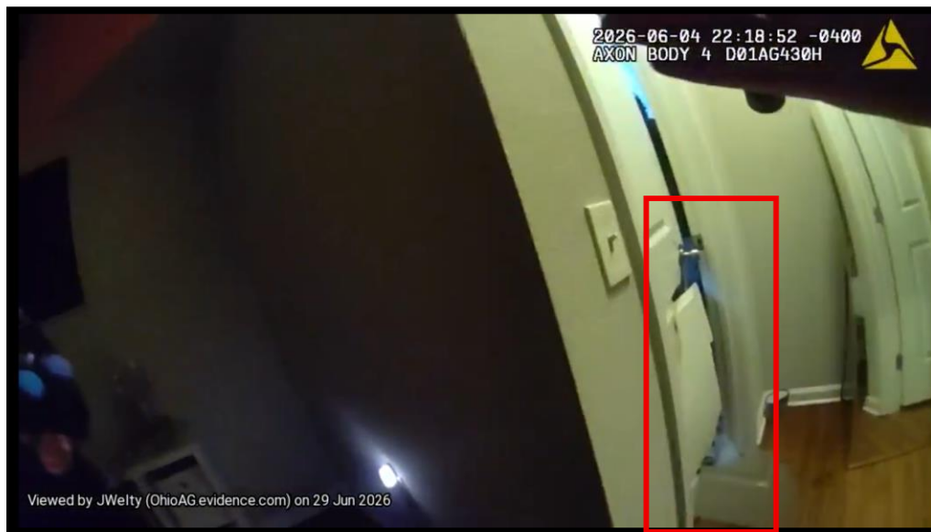
(Figure 3 - Damage visible to the bathroom door)
