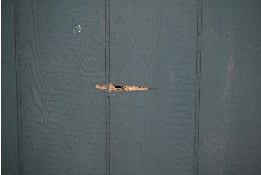
Apparent ballistic impact on west, shed wall
