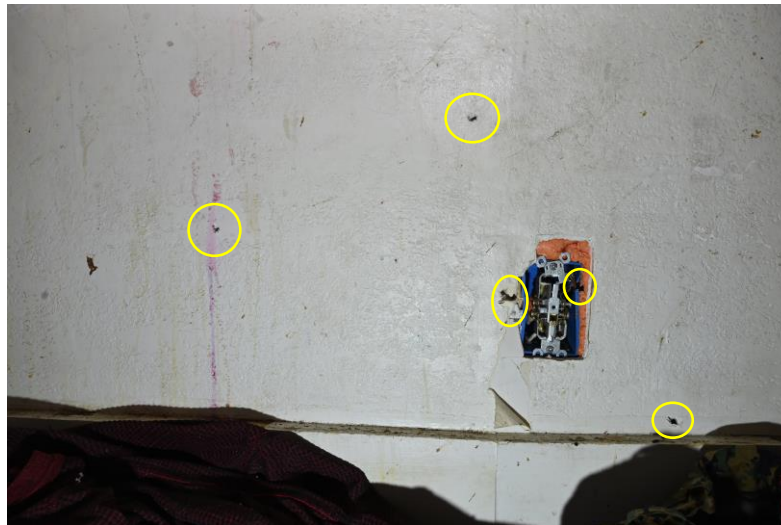
Ballistic impacts on west wall of bedroom
