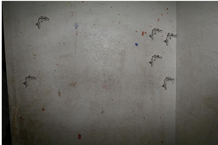
Bullet impacts on interior south wall of bedroom.
