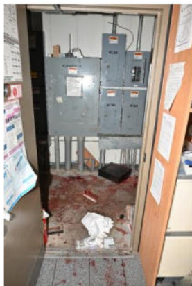
Image #9 – Electrical Room
