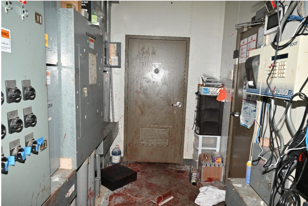
Figure #7 - Electrical room looking at office door (looking west)
