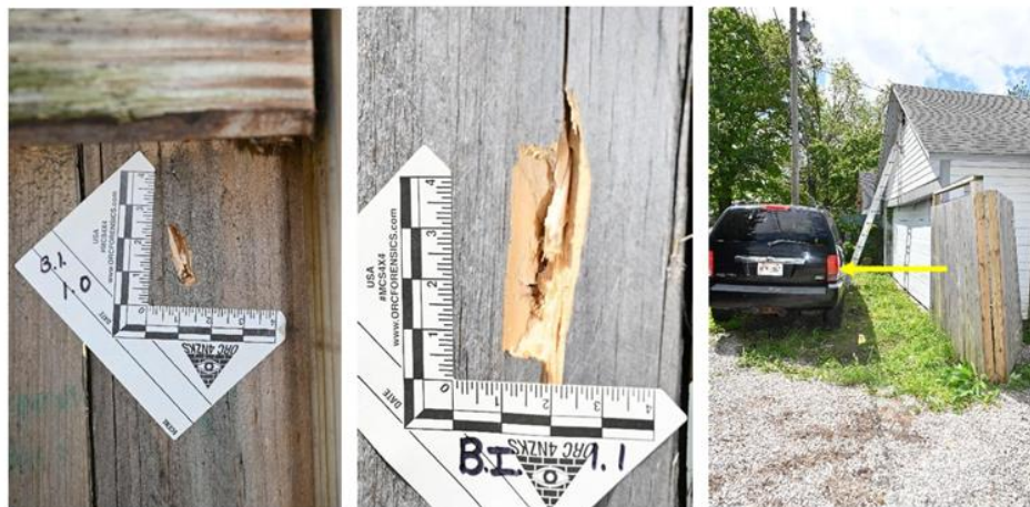
Image #3 – Damage to Fence Near Alley & Fired Bullet
