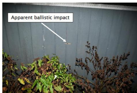
Figure 11 - Ballistic Impact at the back of the shed.
