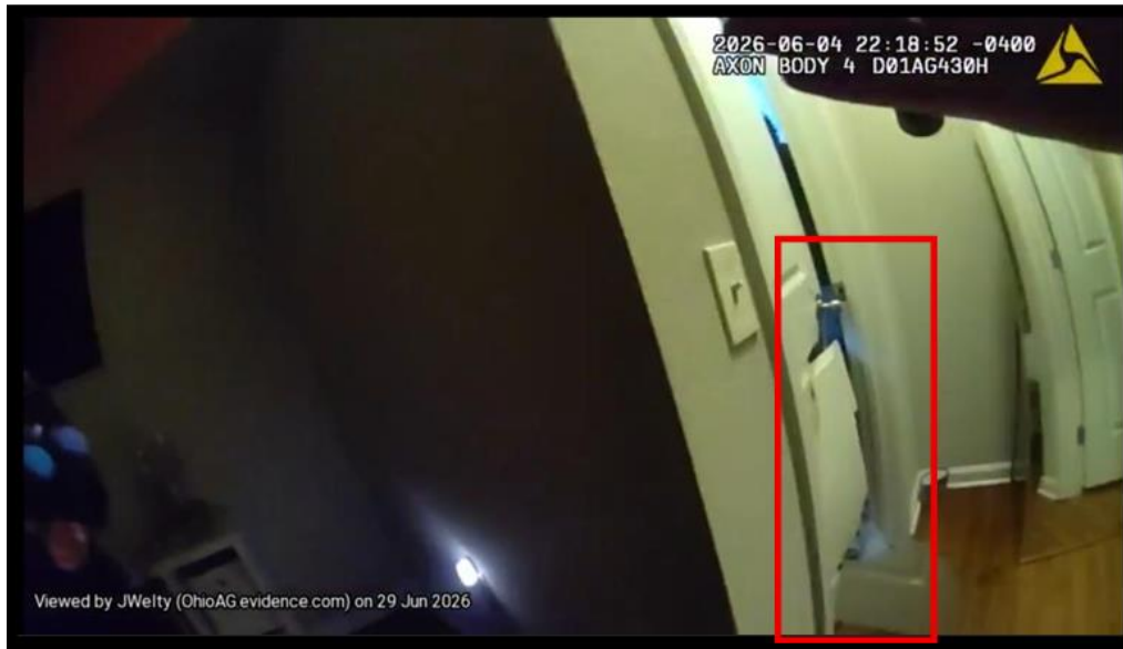
(Figure 3 - Damage visible to the bathroom door)
