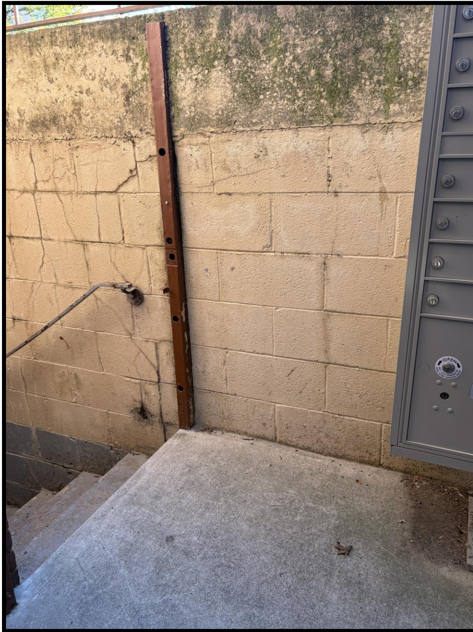
Figure 5: Possible bullet impact marks on east wall
